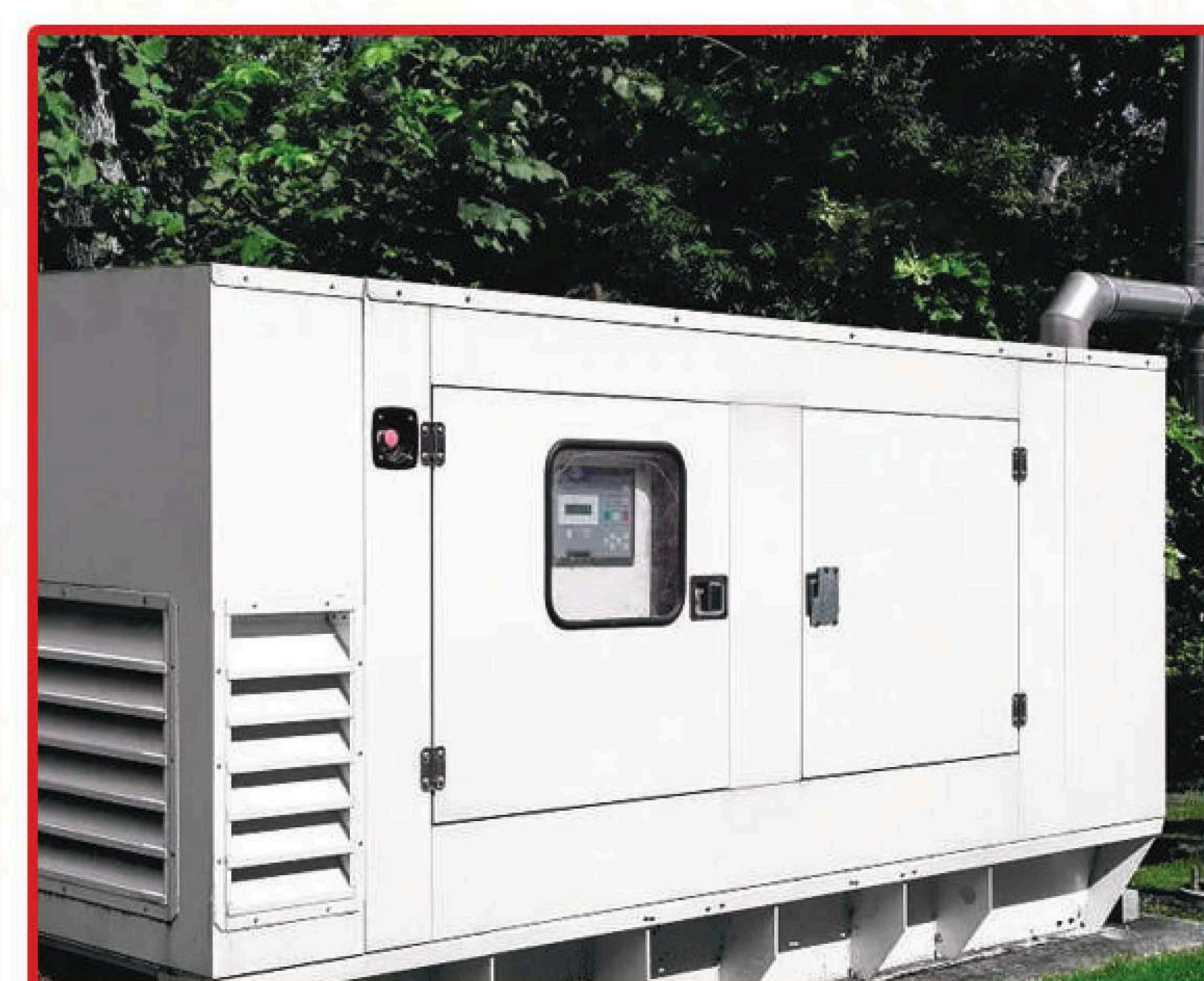
COMMON AREA POWER BACKUP
